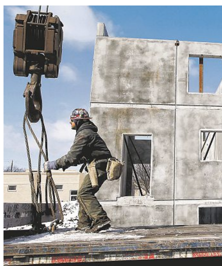
Victor Lunderos of Northwest Steel secures a crane hoist to a prefabricated concrete wall before it is lifted into place.
