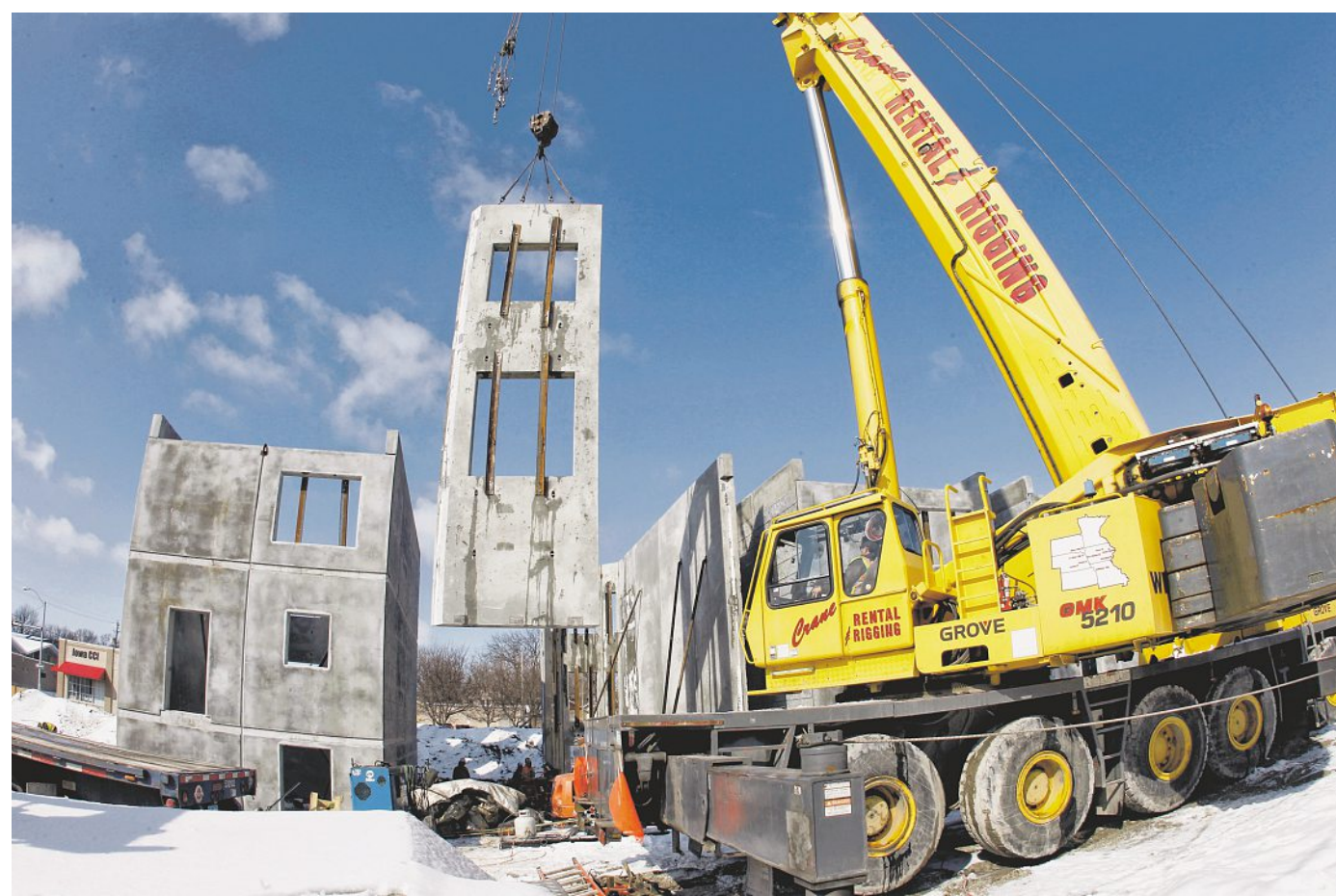
A crane hoists a prefabricated concrete wall at the Greystones construction site at Martin Luther King Jr. Parkway and Forest Avenue on Tuesday. When completed, the project will provide 26 homes for low-income residents. CHRISTOPHER GANNON/REGISTER PHOTOS
